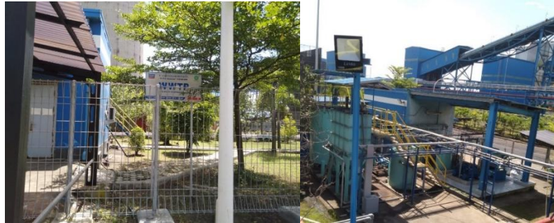
Gambar 2. 2. Waste Water Treatment Plant (WWTP) Unit 1 x 660 MW
