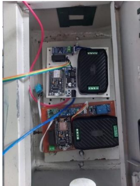
Wiring system dan wiring monitoring
